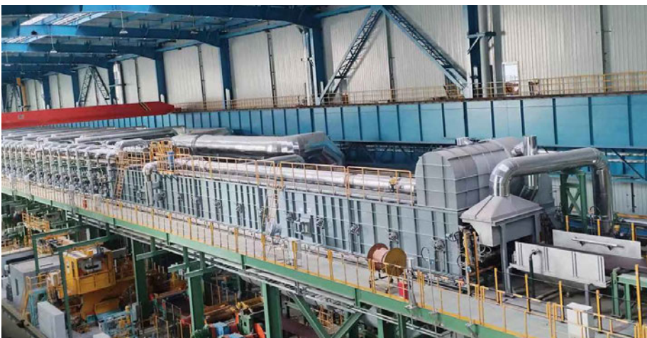
Annealing and pickling line for electrical steel production. (Photo: Fives)
