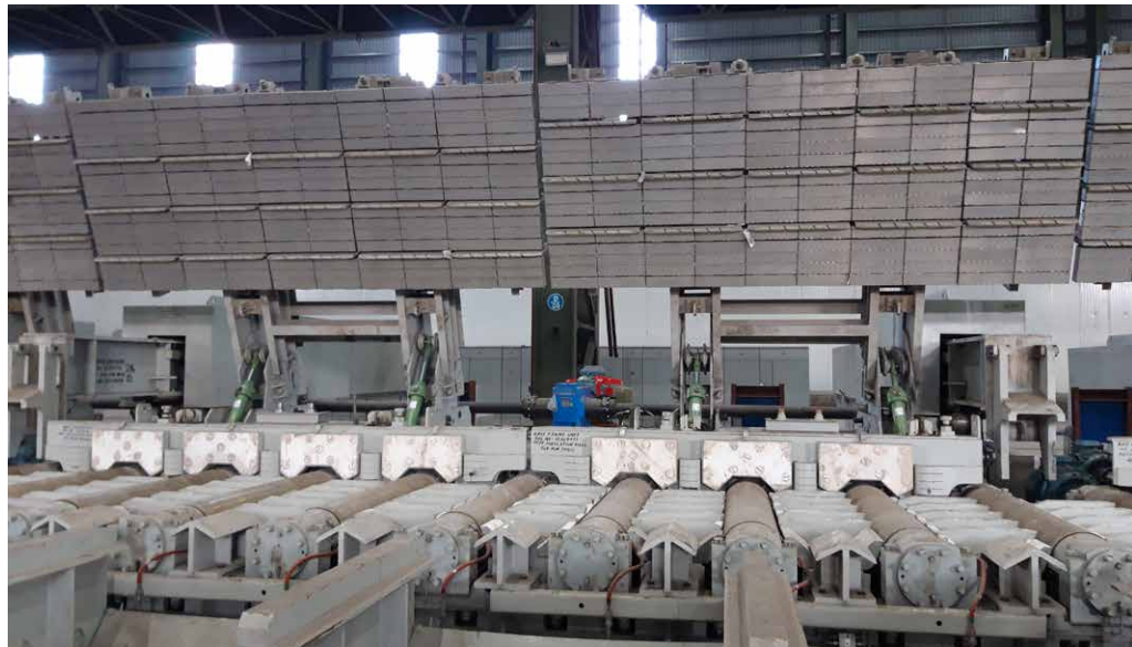
The maintenance friendly modular insulating elements of the HIBOX® heat preservation hoods are mounted on the panels (Picture: SMS group)
