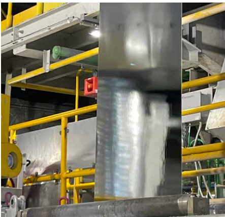
A gloss meter was introduced at the furnace's entrance to measure strip brightness (Picture: Fives)
