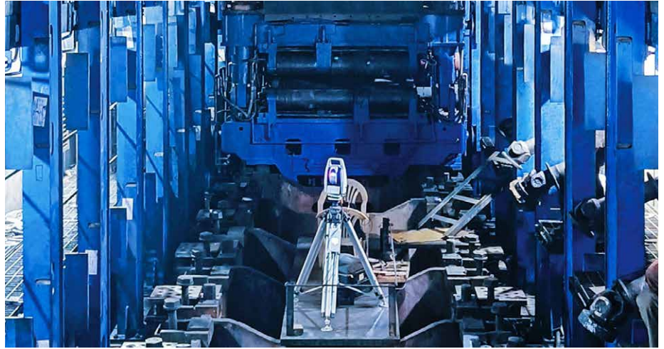
The slab caster at the Bhilai Steel Plant during refurbishment (Photo: Danieli)
