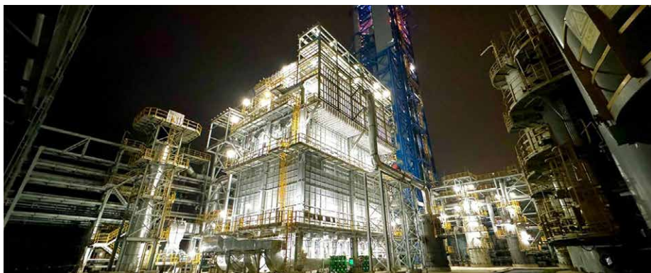
The new DRI plant recently commissioned at Baosteel Zhanjiang Iron & Steel (Photo: Danieli)
