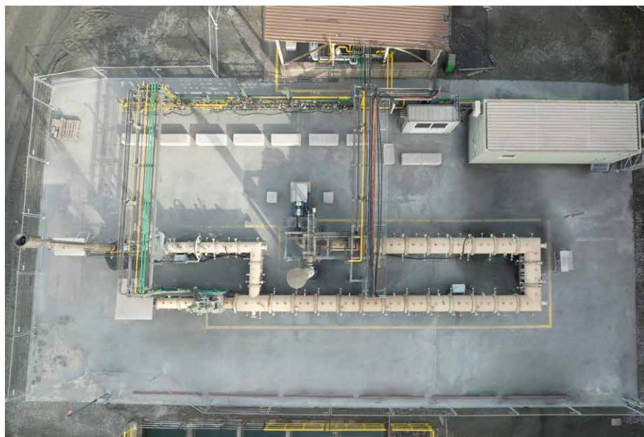
Pilot plant for syngas generation at ROGESA (Picture: SMS group)
