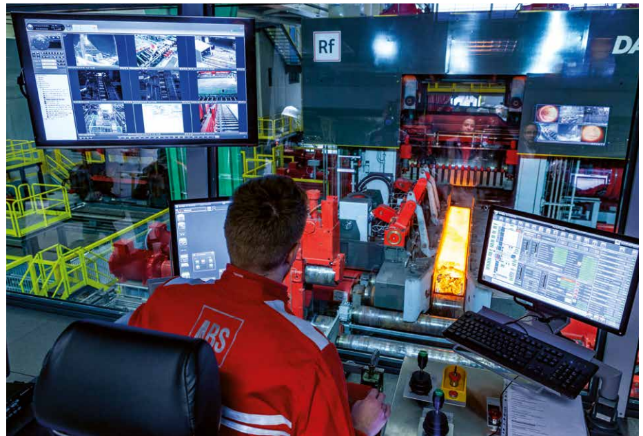
Figure 2. The rolling team can supervise the plant using an advanced operator interface (Picture: Danieli)
