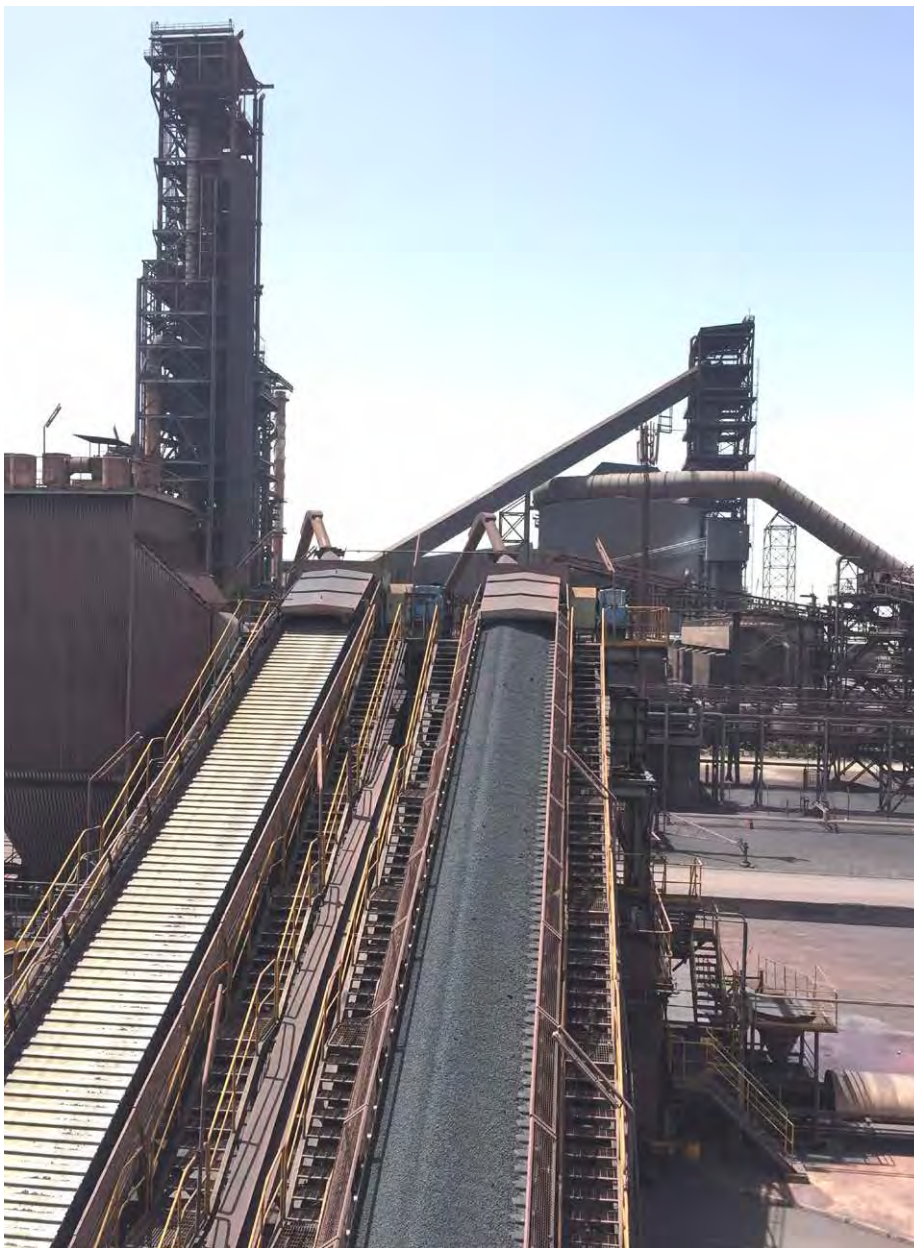
In the foreground, Bahrain Steel Company plant with two pan conveyors type KZB-K for conveying and cooling iron ore pellets at a capacity of up to 1,410 t/hour per conveyor. In the background the steelworks SULB Bahrain with a Midrex direct reduction plant and hot DRI charging (Picture: Aumund)
