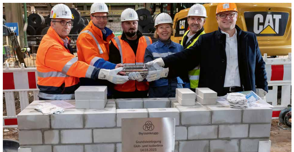
Foundation stone laying for the new annealing and isolating line at thyssenkrupp in Bochum (Photo: thyssenkrupp/GIL)
