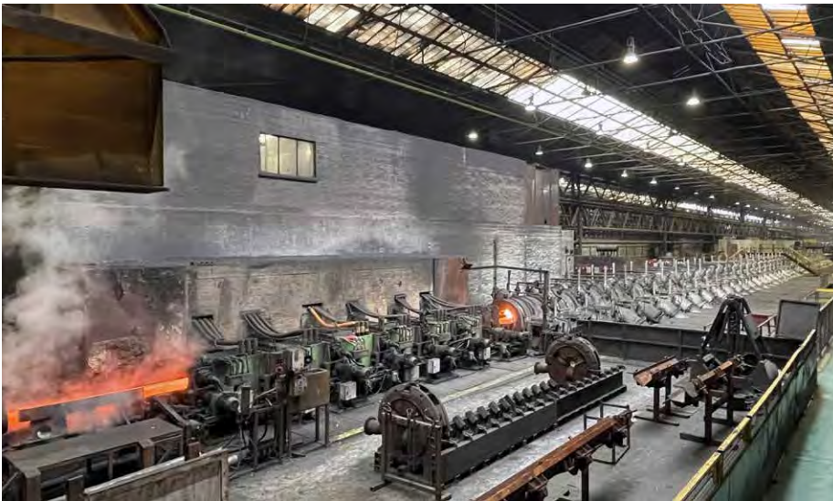
Tata Steel is to upgrade the electric induction furnaces in the stretch reduction mill at its Corby site (Photo: Tata Steel)
