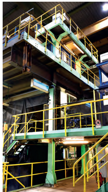
The sensor is arranged in the run-out section of the electrolytic galvanizing line (Picture: thyssenkrupp Steel Europe AG)
