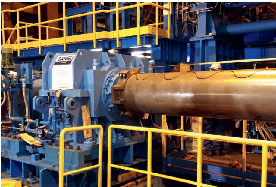
Upgraded entry section of the Mardyck pickling line (Photo: Danieli)
