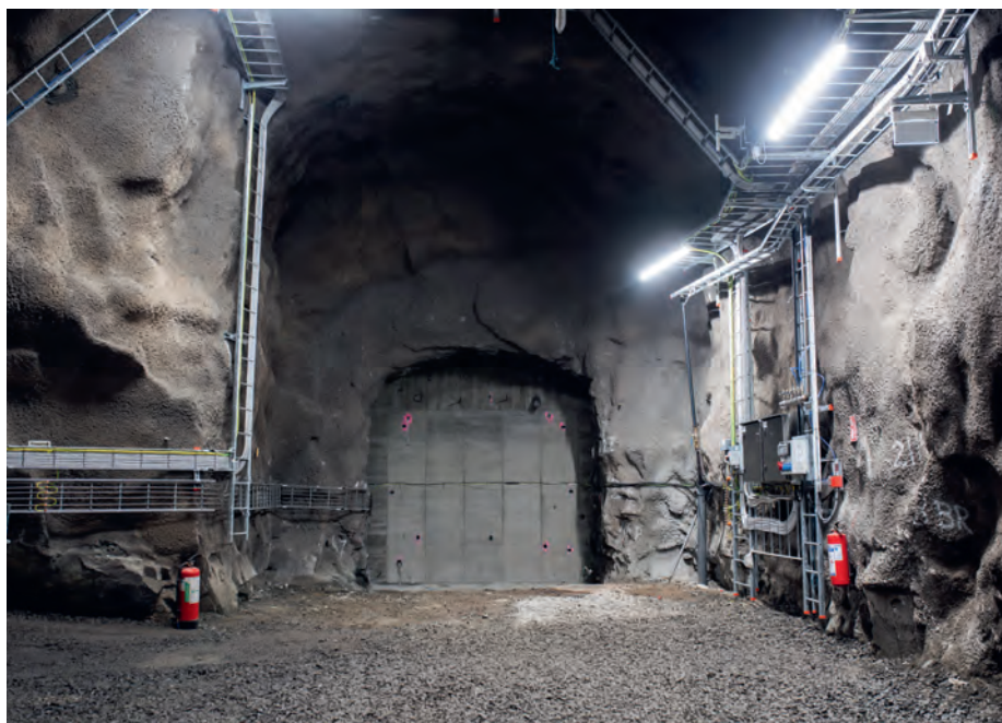
Hybrit cavern for storage of fossil-free hydrogen gas (Photo: SSAB)
