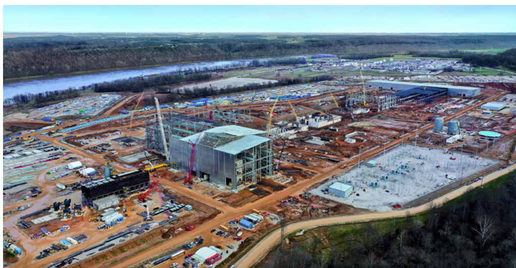
Aerial view of the Nucor Brandenburg construction site in January 2022 (Picture: Danieli)
