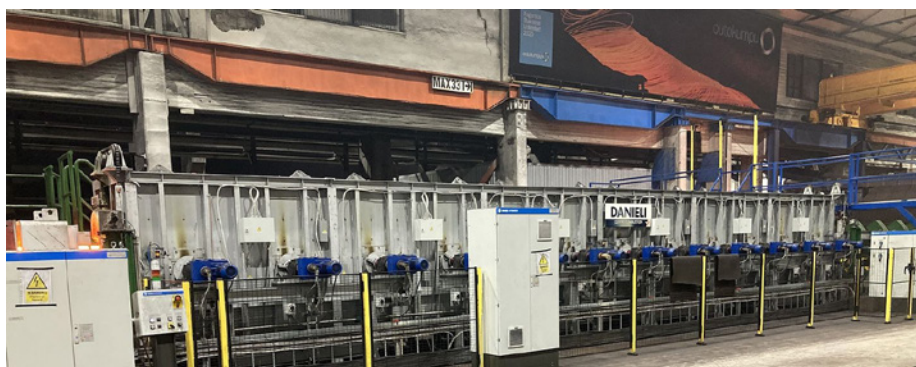
The new soaking furnaces at Fagersta Stainless in Sweden (Photo: Danieli)
