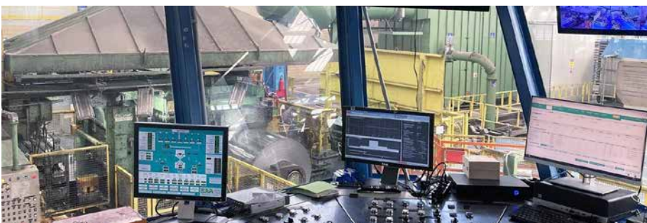
State-of-the-art control room in a cold rolling mill (Picture: Danieli)
