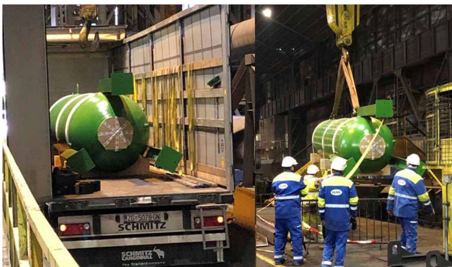
For the modernization of the descaler, new accumulators have been installed (Picture: NLMK)
