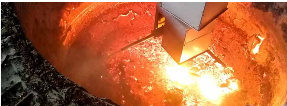
For the gunning repair, the gunning manipulator is set from top down into the EAF (Picture: VELCO)
