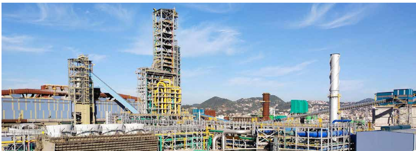
The new Midrex plant has a rated production capacity of 2.5 million t/year (Picture: Midrex Technologies)
