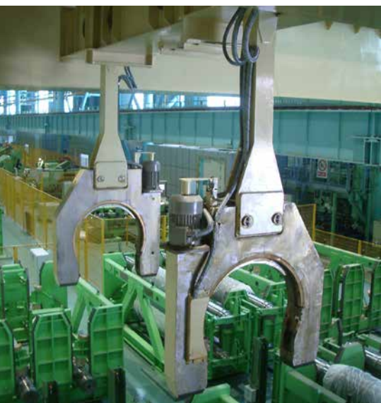
View of an automated roll shop (Picture: Tenova)
