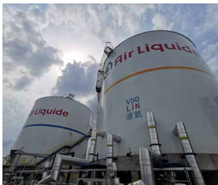
Existing air separation units in China (Picture: Air Liquide)
