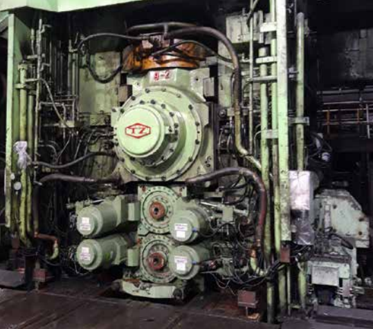
One of the finishing mill stands of Benxi Iron & Steel's hot strip mill after the revamp (Picture: SMS group)
