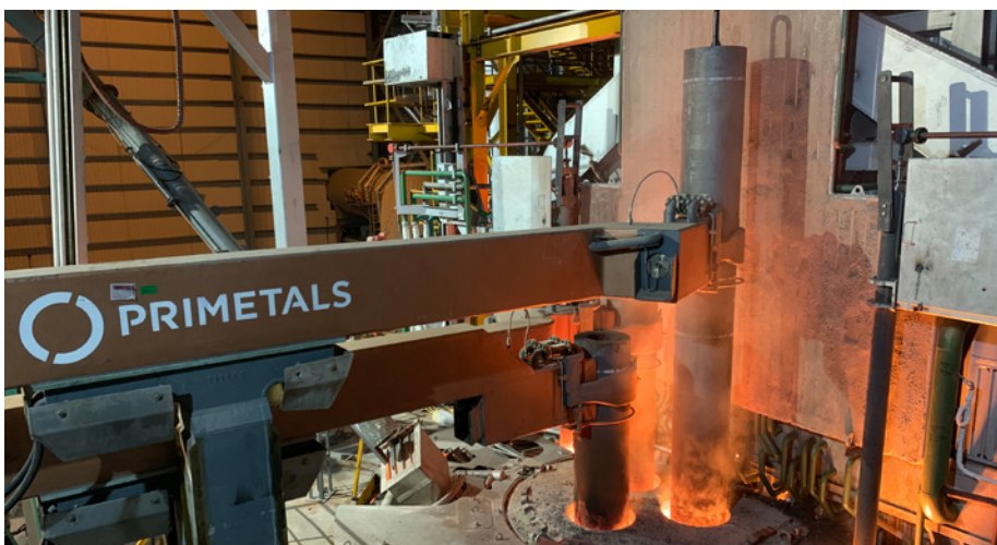
Roof with electrodes of the EAF Quantum furnace (Picture: Primetals Technologies)
