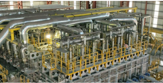
Walking-beam reheating furnace for billets (Picture: Danieli)
