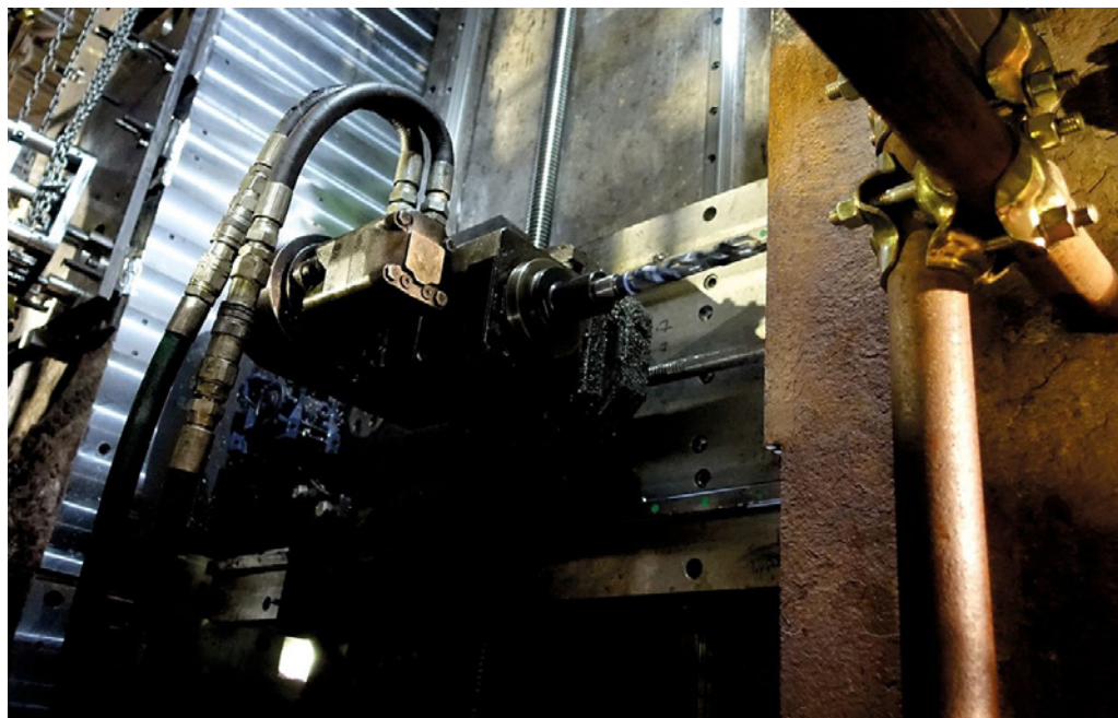
Refurbishment of the mill housing in the Marcegaglia plate mill (Picture: Danieli)
