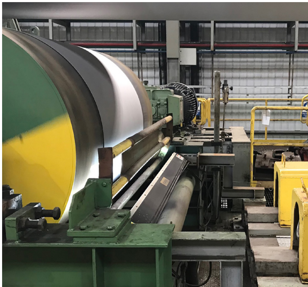
At Ternium Pesqueria plant in Monterrey, four cameras, two each side, are installed in bright field mode just after the pickling process. (Picture: Ternium)
