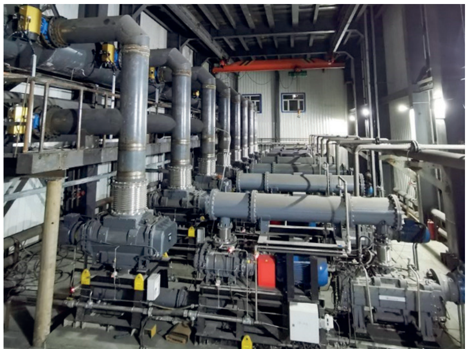
Figure 9. Smart pump configuration. VD/VOD application with mechanical vacuum dry pumps – plant G (2020) (Picture: Danieli)
