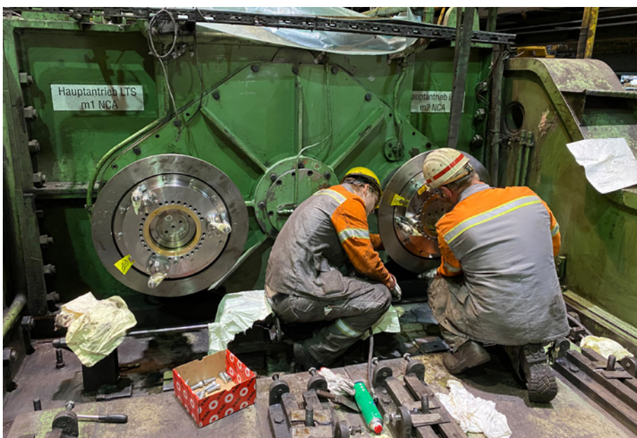
The shear drive was retrofitted with the new self-reset torque limiter in May 2020 (Picture: Malmedie)
