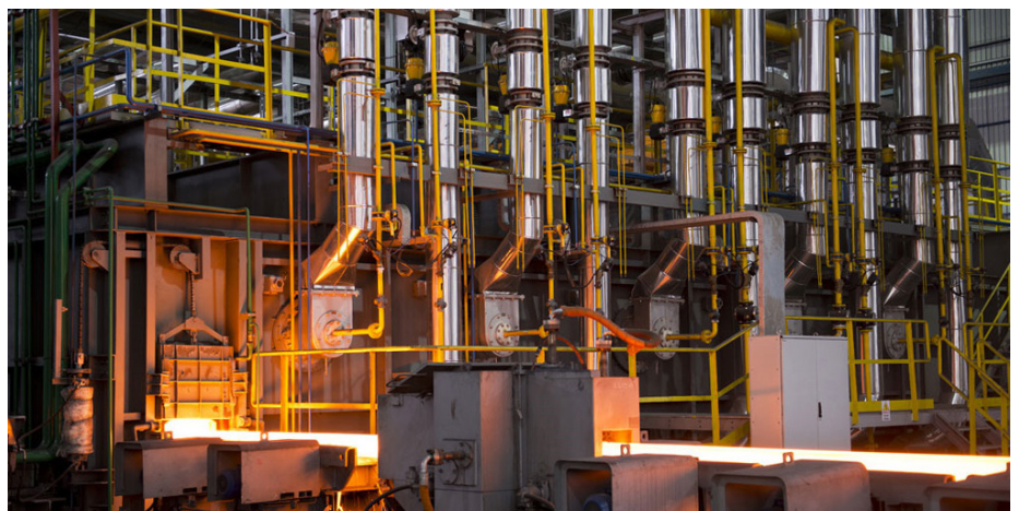
The discharge end of a reheating furnace from Fives in operation (Picture: Fives)
