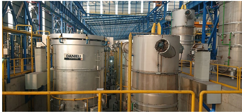
New bell annealing furnaces installed at Atakas in Iskenderun (Picture: Danieli)
