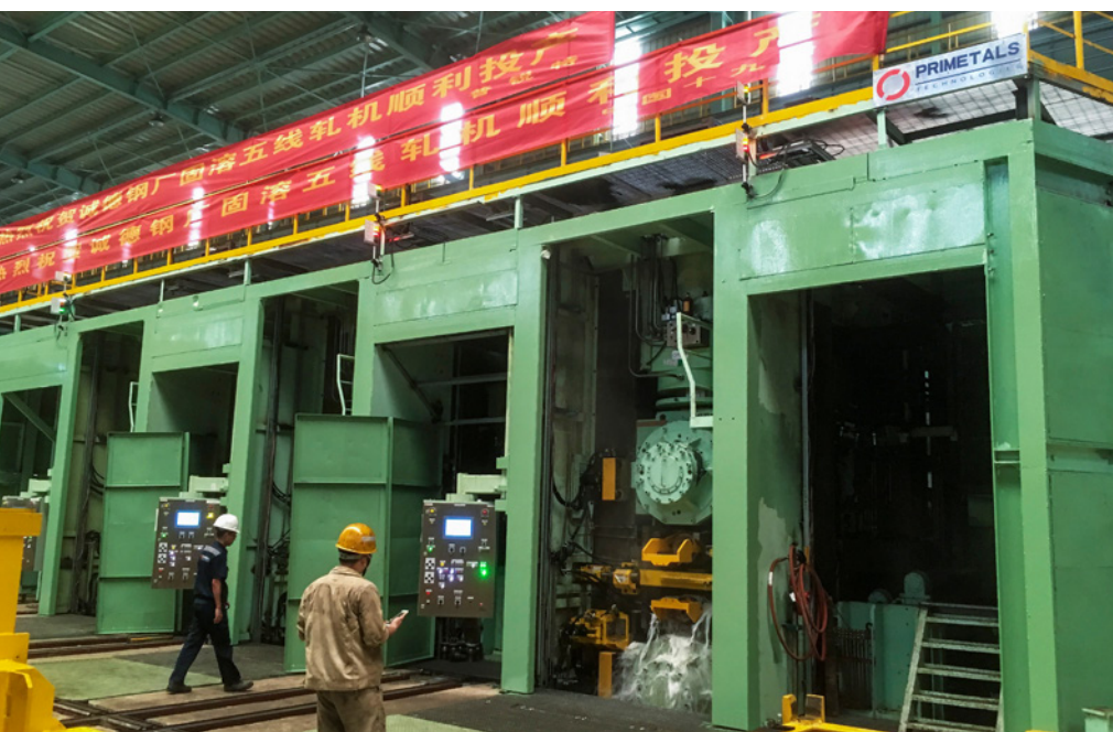
Six months from the rolling mill start-up, Beihai Chengde awarded the PAC for the 3-stand Power X-HI continuous tandem cold mill (Picture: Primetals Technologies)
