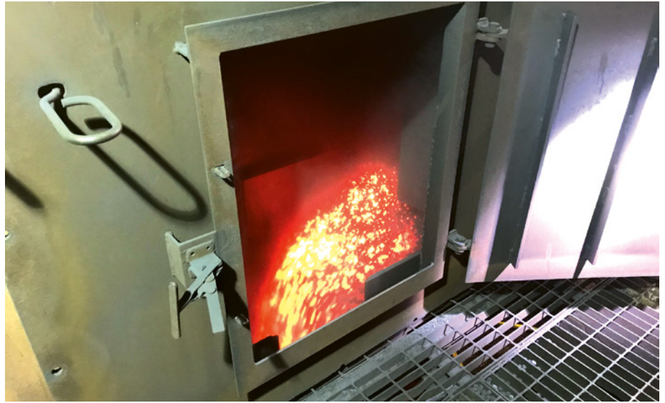
At Grange Resources, the new steel plate conveyor will transport iron ore pellets at a temperature of up to 750°C to the cooler (Picture: Aumund Fördertechnik)
