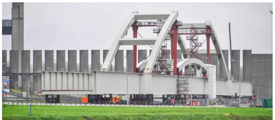
The assembly of the various sections on the assembly area close to the final site (Picture: Hollandia Infra)
