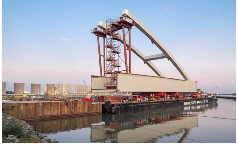
The combination segment of eastern bridge deck and arch section upon arrival at the assembly site (Picture: Hollandia Infra)
