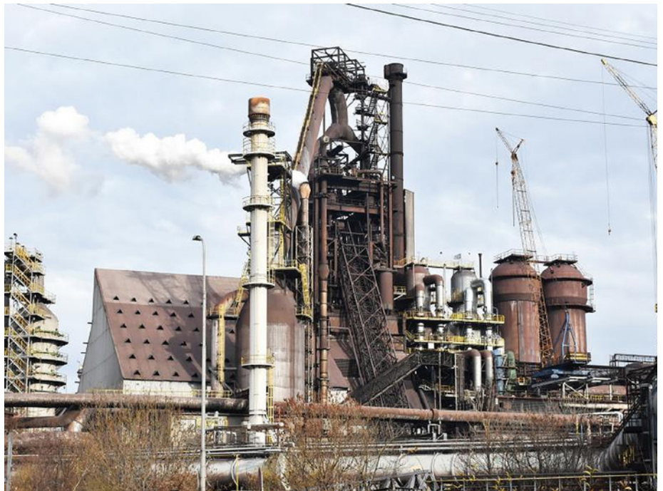
The third new hot blast stove commenced operations in November 2019 (Picture: Trinec Iron and Steel Works)
