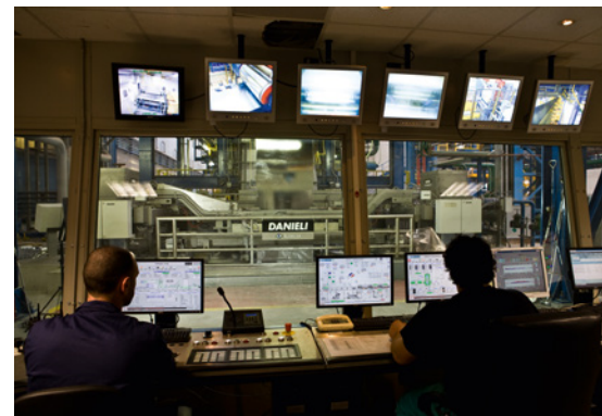
Figure 7. Danieli Automation (DA) system allows the complete control by operators with detailed diagnostic capability (Picture: Danieli)
