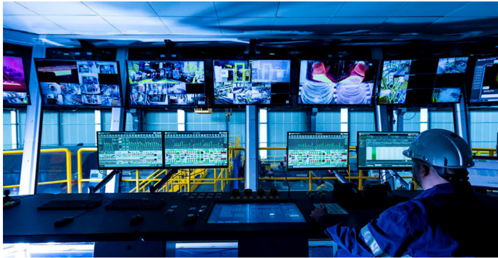
Control room of the extended wirerod mill (Picture: Danieli)
