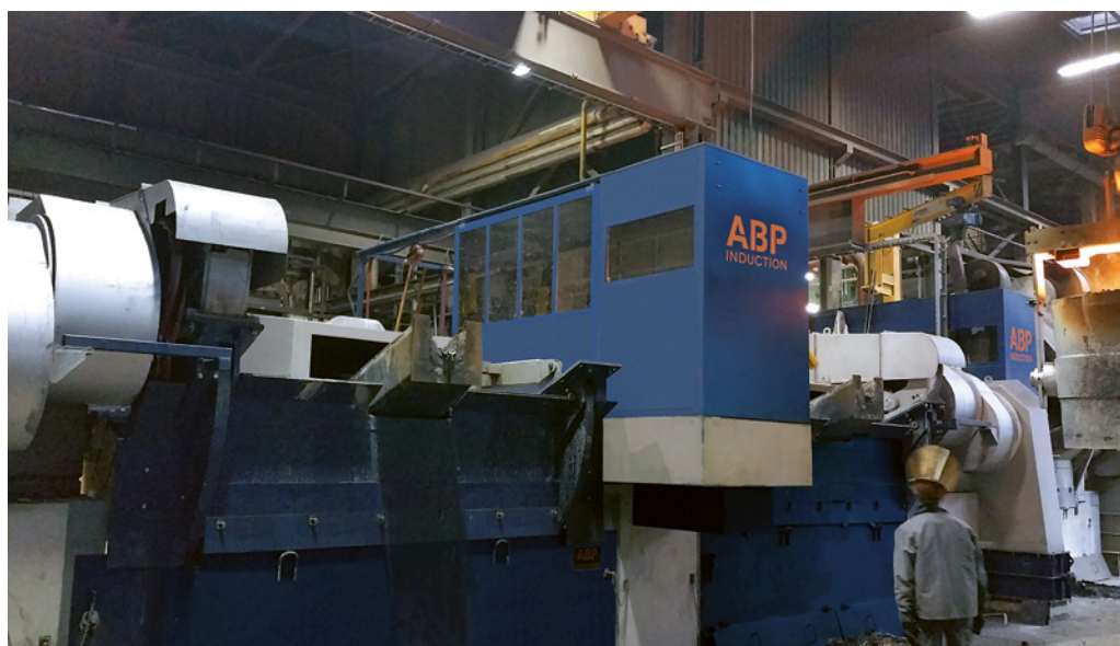
Induction melting furnace IFM 7 Twin Power from ABP, capacity 13.4 tons, rated power 6 MW (Picture: ABP Induction Systems)
