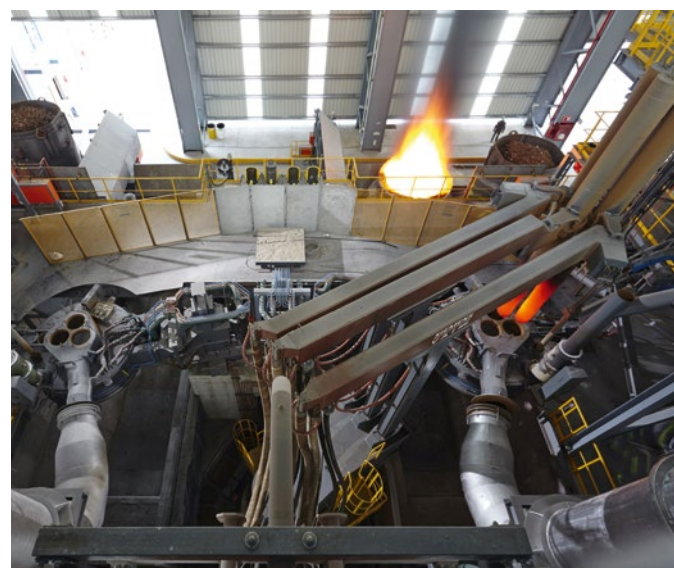
Twin ladle furnace in operation (Picture: Primetals Technologies)
