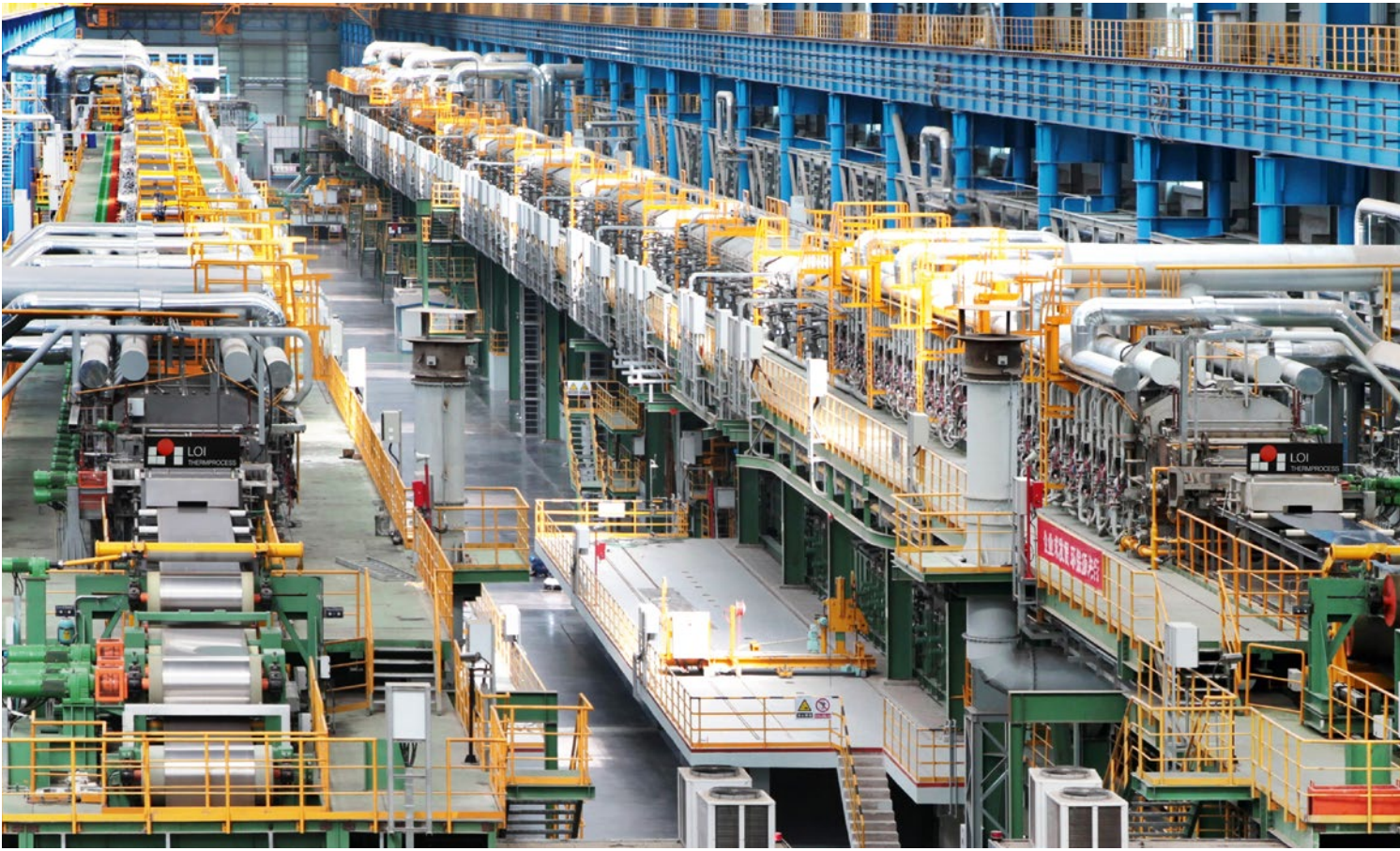
Two DCL-Lines for grain oriented electrical steel installed at Shougang Qian'an, China (Picture: Tenova LOI Thermprocess)
